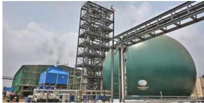
Energy security: The compressed biogas plant at Brahmapuram currently processes about 50 tonne of biodegradable waste a day.
