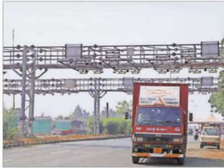
The MLFF system works without a boom barrier and vehicles are not supposed to stop for toll payment. EXPRESS
