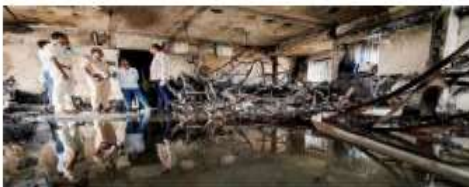
Shared walls: Police personnel conducting an inspection after a fire broke out at Kabaja Residency in MUM Complex, in Vashi, Navi Mumbai, early on Tuesday.
