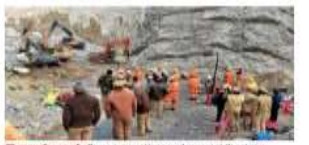
Through search rescue operations under way at the stone quarry in Sonbhadra district, Uttar Pradesh. > PAGE 10
