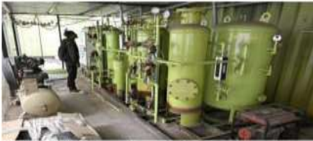
A biogas plant at the Waste-to-Energy unit in Karamangala in Bengaluru. A. Srinivasan
