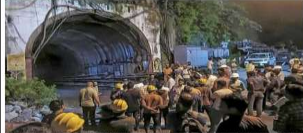
Trapped underground: Rescue workers gather after water and debris entered an under-construction tunnel in Piplodhi near Channarayana in Hyderabad on Thursday. Six workers are feared trapped in the tunnel. Photograph by Ravi K.
