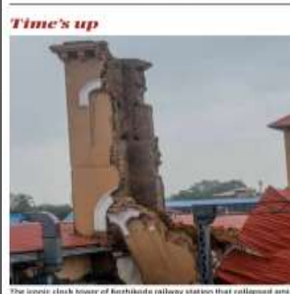
The iconic clock tower of Bangladesh railway station that collapsed amid heavy rain on Thursday. It was set for a controlled demolition later in the day after developing cracks recently. » SOURCE: AP/WIDE WORLD
