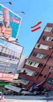
On edge: A building damaged in a 7.4 magnitude earthquake that struck east Taiwan on Wednesday. Nine people were killed and over 1,000 injured. The toll was relatively low owing to the nation's high levels of quake preparedness, say experts. AFP (REPORT ON PAGE 14)
