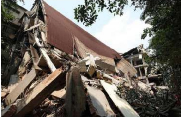
Crumbled blocks: A damaged building in New Taipei City, after a major earthquake hit Taiwan's east on Wednesday. AFP
