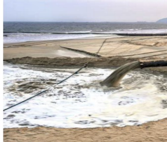
Checking erosion: The extended beach formed after six weeks of sand pumping as part of the beach nourishment work by Dredging Corporation of India in Visakhapatnam on Monday. K.R. DEEPAK
