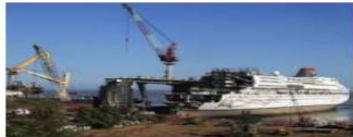
More on the decks: The additional plots can double the ship-recycling capacity of Alang to 9 million LDT, the venue
