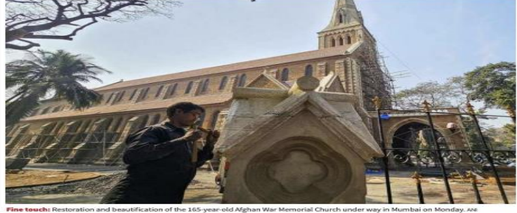
Fine touch: Restoration and beautification of the 165-year-old Afghan War Memorial Church under way in Mumbai on Monday. ANI
