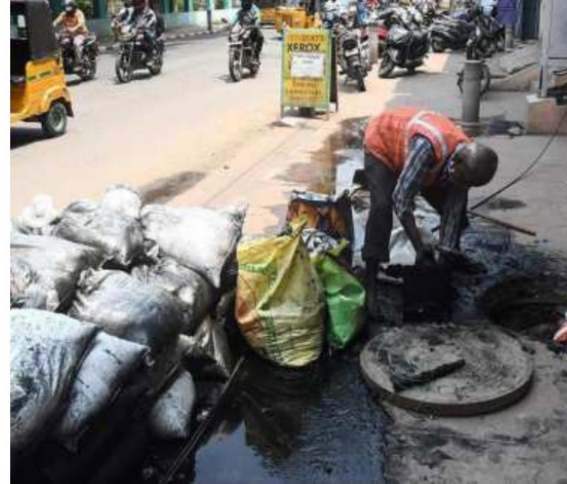
In the deep: Senior Ministry officials have differentiated manual scavenging from hazardous cleaning of sewers. FILE PHOTO
