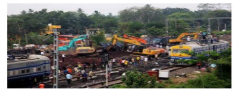
Fast-paced work: Workers busy restoring the track at the accident spot at the Bahanaga railway station in Balasore district of Odisha on Sunday. SHIVANJAN ROUT
