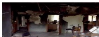
Deceptive attacks: A building damaged in the alleged incursion in the Belgorod region of Russia on Monday. AP
