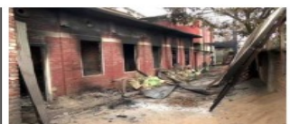
Conflict zone: The charred remains of houses days after violent clashes in Manipur. The unofficial death toll is over 50,000.
